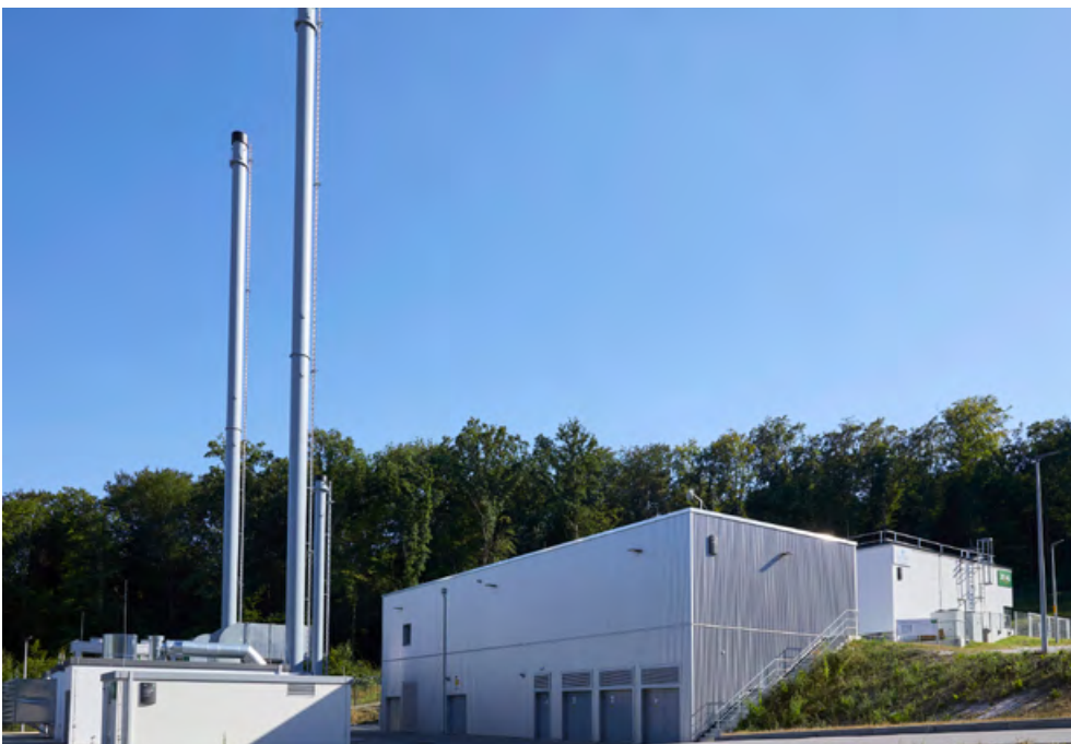
The green hydrogen, produced by the H 2 ORIZON facility is processed, compressed and directly filled into special transport vehicles for distribution. Copyright: DLR Lampoldshausen
